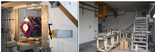
Figure 5: start of the assembly of equipments at GANIL/SPIRAL2. Left: first quadrupole installed, right: beginning of the assembly of the mechanical frame.
