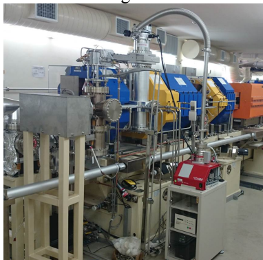
Figure 7: The exhaust pumping system in TPS storage ring.
