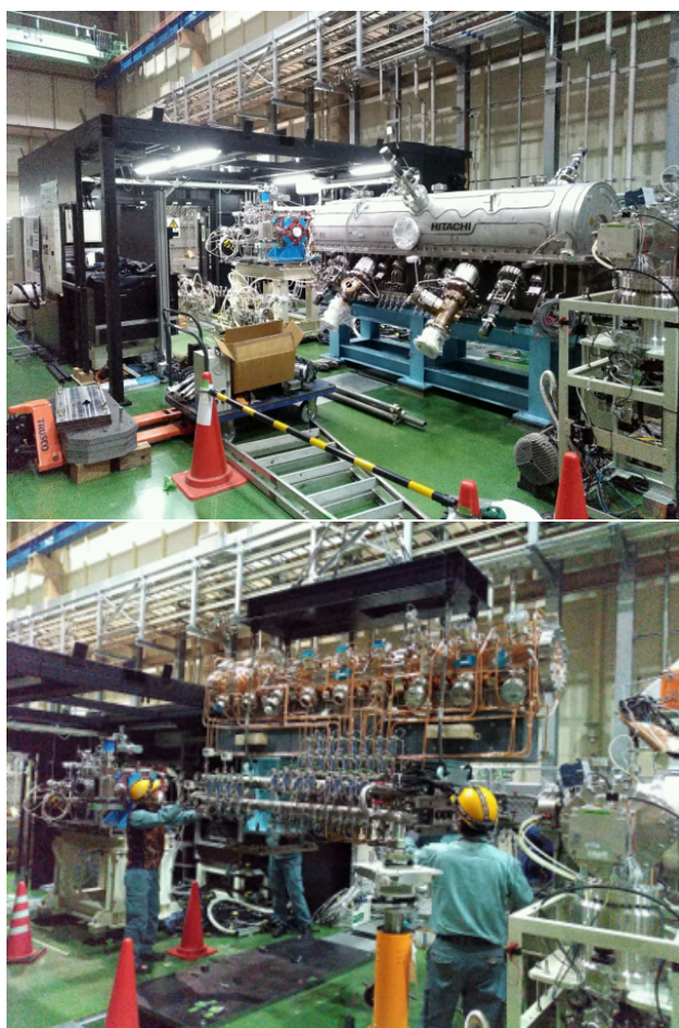
Figure 2: Decommissioning of RFQ I (upper) and installation of the new RFQ (lower).
