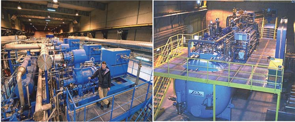
Fig. 8.12. Cryogenic plant providing 18 kW @ 4.5 K. Left: compressor station. Right: cold box.
