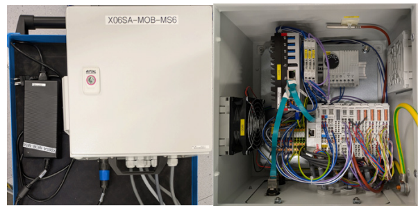
Figure 13: Portable control box.
