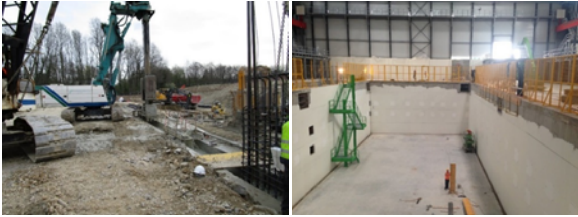
Figure 38: Photographs taken during (left) and after (right) diaphragm walling works at CENF.
