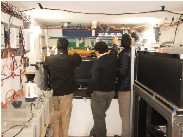
(a) The CRLF Ready for Laser installation
