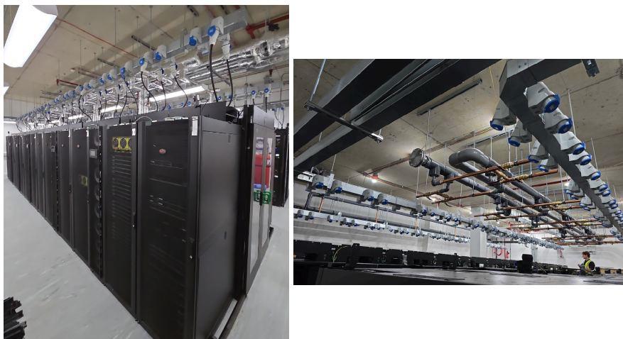
Figure 2. Pictures of the actual data centre, showing the racks, in row coolers, water cooling circuit and room infrastructure (light and power)
