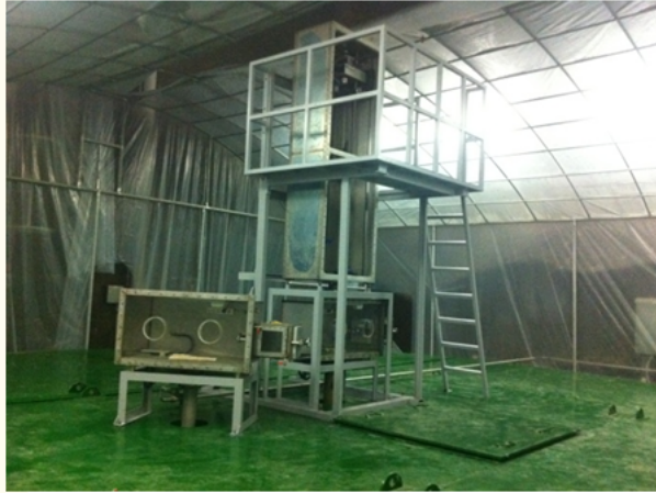
Figure 4.3: Installed 3D system. Two installed 1D system is also shown.
