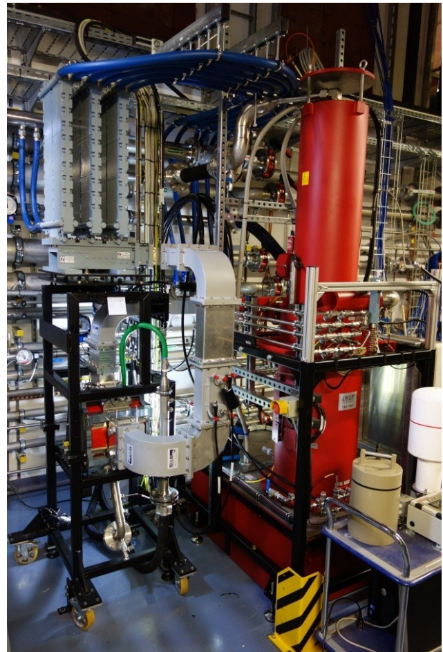
Figure 4: Installed klystron with circulator (left bottom) and 300 kW waterload (left top).
