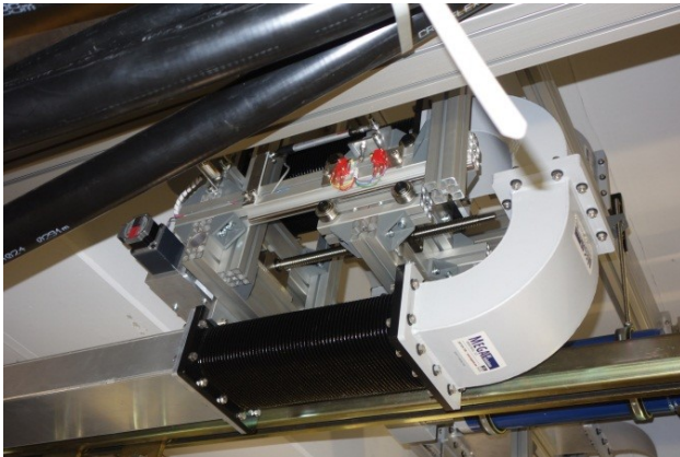
Figure 6: Motor actuated waveguide phase shifter.
