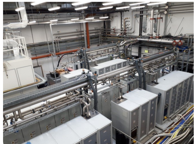
Figure 2: Klystron power supplies. Each power supply consists of two cabinets 32.6 kV 9.2 A, one combining cabinet and one rack for mains and controls.
