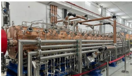
Figure 4: HIAF RFQ have been installed and commissioned.
