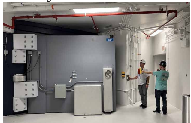
Figure 13: Massive concrete-filled Target Bay doors are opened after a high-yield experiment, under stringent radiation survey protocols.
