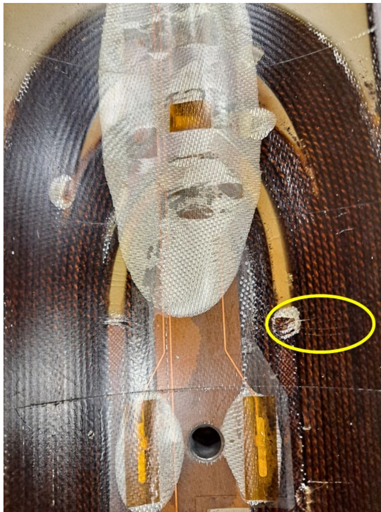
Figure 6.2: detail of coil 214 Lead End. The yellow box shows the position of “scratches” starting from the wedge to end-spacer transition
