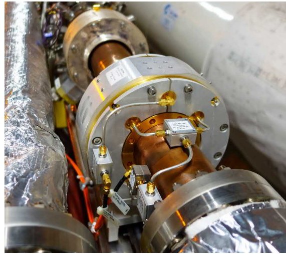
Figure 4.18: WCT R2B installed in the measurement position.
