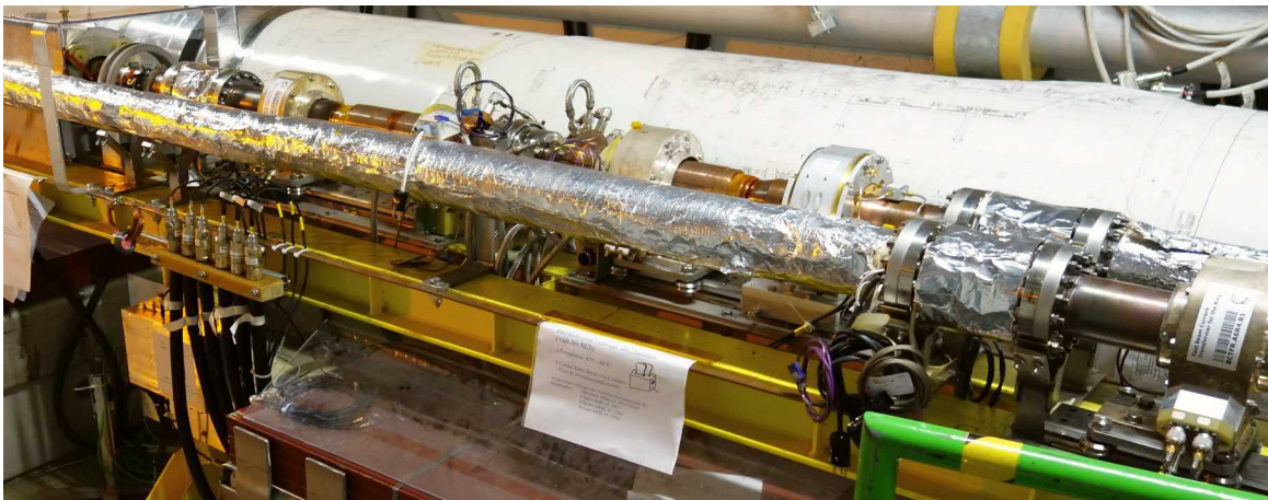
Figure 4.19: WCT R2B with its head amplifier fixed to a yellow vertical support next to FBCT R2A. One of the DCCTs can be seen under the transparent plastic cover.
