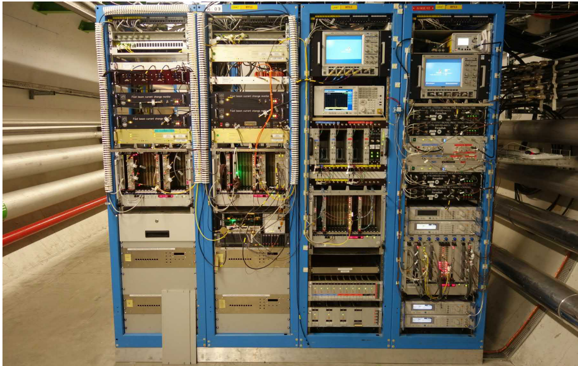
Figure 4.27: 19-inch racks hosting the WCT, FBCT and ICT acquisition electronics.
