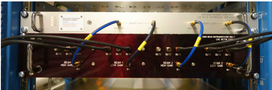
Figure 4.26: Distribution amplifier and a box common-mode chokes installed in a 19-inch rack.
