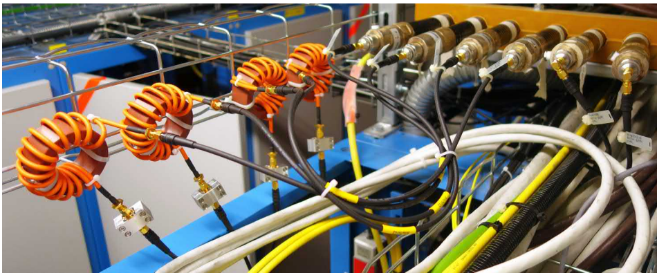
Figure 4.25: Common-mode chokes and 200 MHz low-pass filters installed at the end of the Heliac coax cables before the distribution amplifier.
