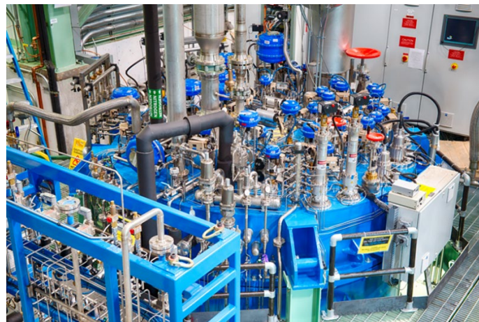
Figure 3: Industrial Cryoplant at Fermilab’s Cryomodule Test Facility
