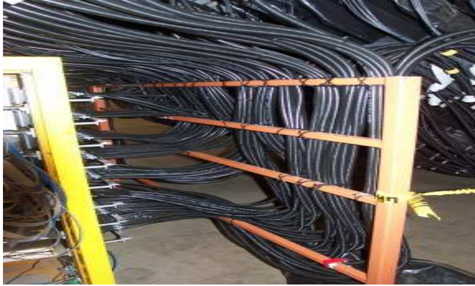
Figure 4.5: Fiber optic cables running from the modules to the steel boxes.
