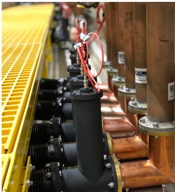
Figure 4: Mega bias tees installed in FRIB.
