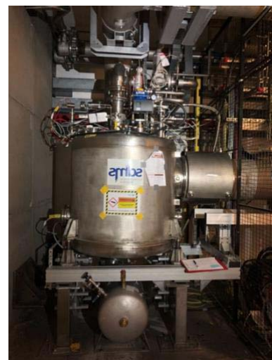
Figure 12: As-built endbox with modifications
