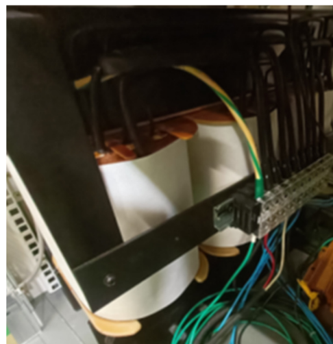
Figure 6: Photo of the transformer stand.
