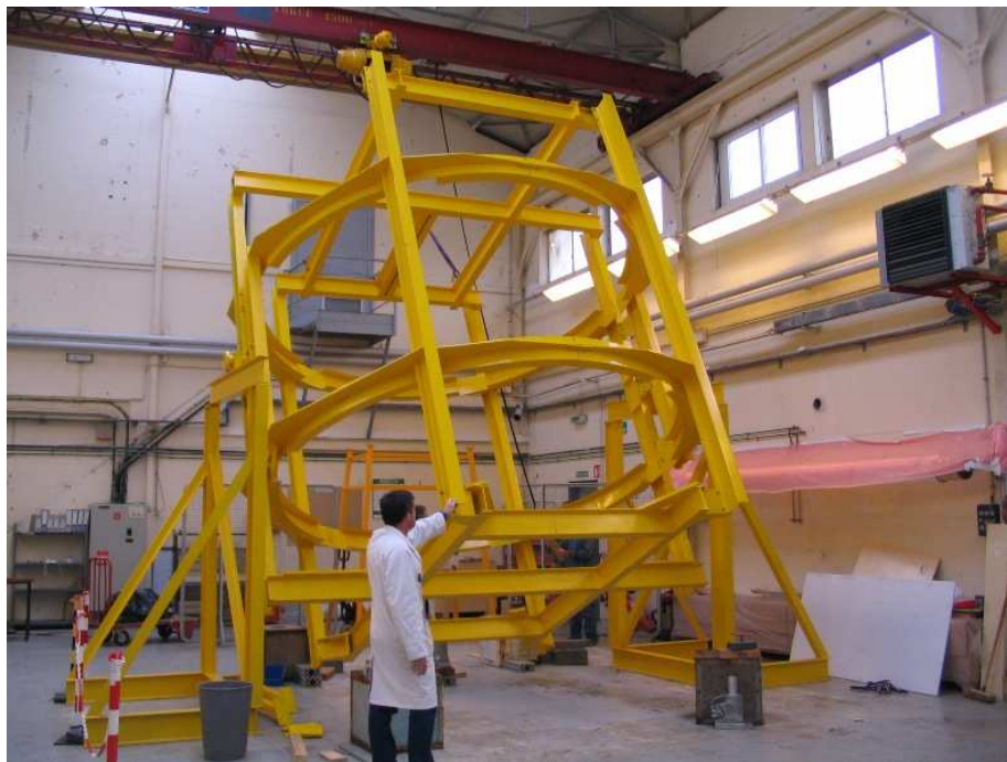
Figure 6. Mechanical tool for the construction, transportation and installation of the \gamma -catcher vessel in the Chooz pit.
