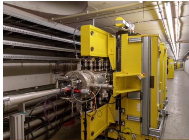
Figure 1: The first in-vacuum undulator in PETRA III.
