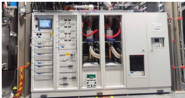
Figure 4: Rack layout of RFPS with cabinet panels on rack III and IV removed
