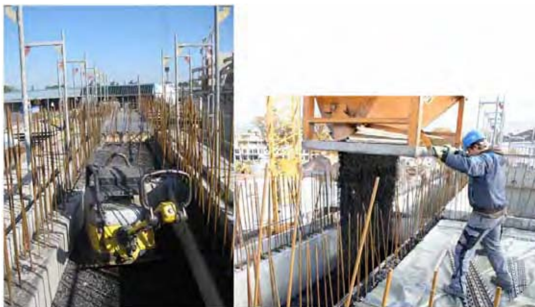
Figure 15: Filling the walls and compacting the material. Using magnetite and EAS (electro arc slag) densities of the mixture up to 3,9 \text{ t/m}^3 can be achieved.
