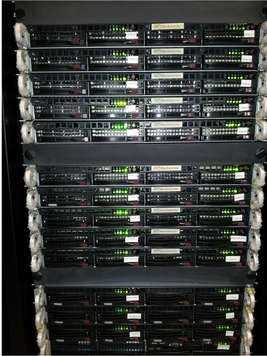
Figure 4.13: The NDOS DAQ Cluster. The cluster takes up half of one computing rack. The ND cluster is similar in size, and the FD cluster is spread over 9 racks.
