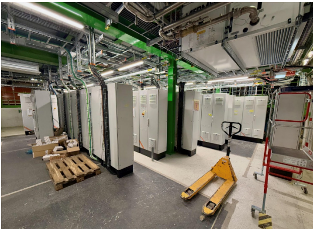
Figure 5: CMS underground control cabinets.
