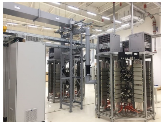
Figure 1: SSA towers of the storage ring RF plant.
