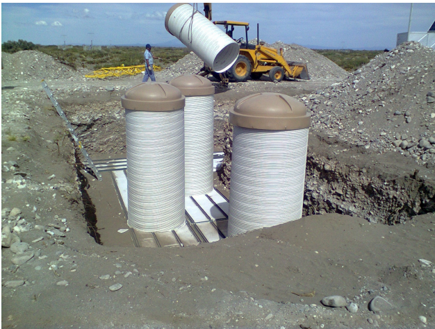
Fig. 3: Deployment of the first twin at Kathy-Turner when installing the service-tubes right before burying the modules.
