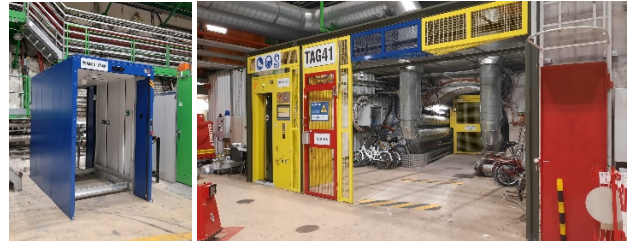
Figure 4: On the left, the MAD, removed, on the right, the access point without MAD.
