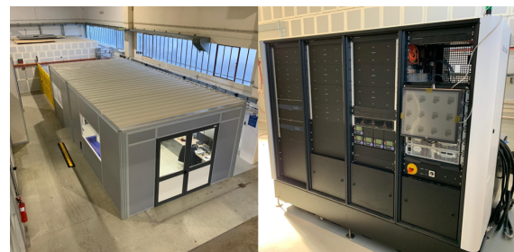
Figure 2: Pictures of the TEX control room, klystron area and bunker (left) and RF power station (right).
