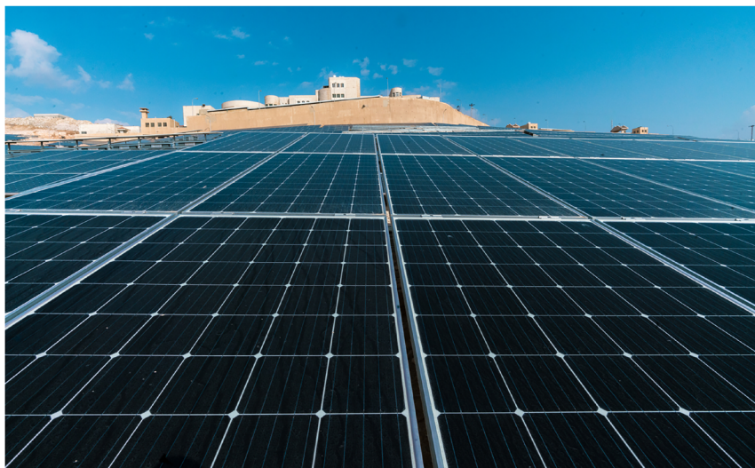
Figure 7. SESAME's solar plant. Photo credit: Noemi Caraban Gonzalez, CERN.
