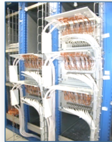
Figure 3. Rack with Front-End Readout Link boards.
