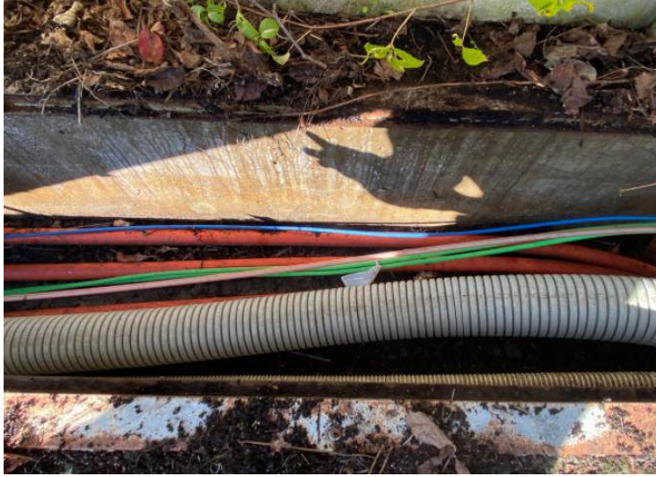
Figure 3.3: Installation conditions of the optical fibers. Two fiber bundles (green sheath) are laid together with the three phases of an MV line (three red coaxial cables). The photo was taken near the receiving substation.
