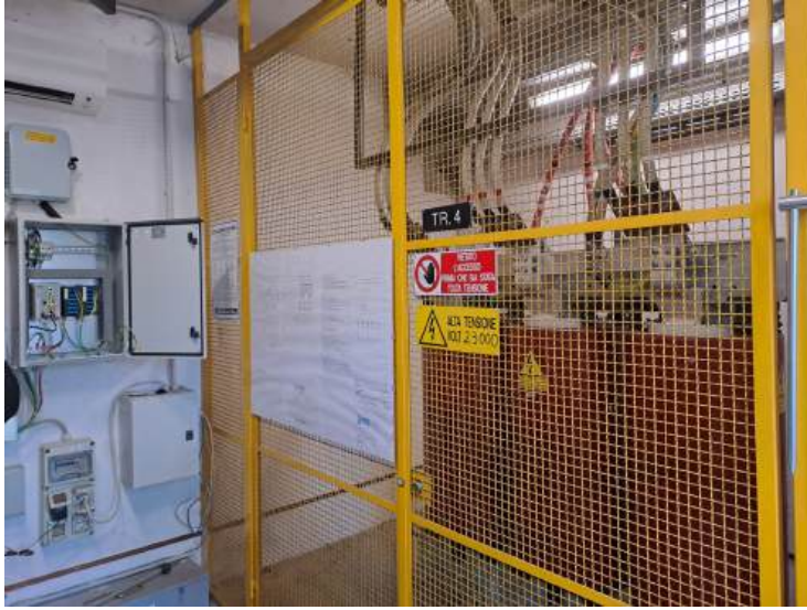
Figure 3.5: Substation B2A. A 23 kV/0.4 kV, 800 kVA MV/LV resin transformer is visible, and on the left the fiber connection panel.
