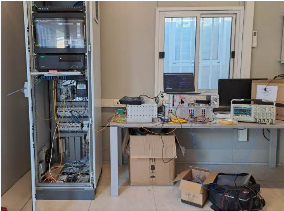
Figure 3.4: Control room of the RSE test facility. The equipment is arranged on the bench. On the left, two stacked boxes can be seen: the lower one contains the optical components, while the upper one houses the laser and RF electronics. In the center, just below the laptop, is the electronics for signal acquisition and processing.
